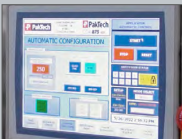
Allen Bradley PanelView HMI
