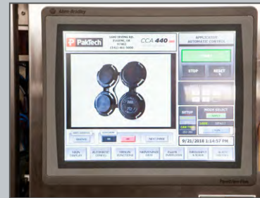
Allen Bradley Panel View HMI
