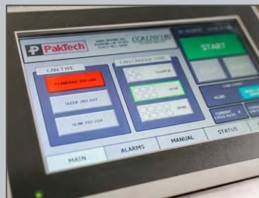
HMI Touch Screen, Status & Alarm Messaging, I/O Status
